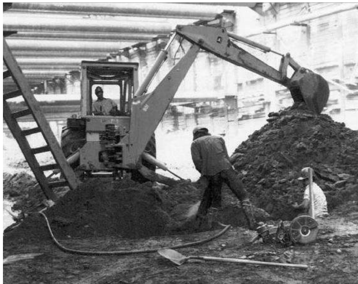
Figure 5.3 Braced cut in the construction of Washington, D.C. Metro, May 1974 (Courtesy of Ralph B. Peck)
