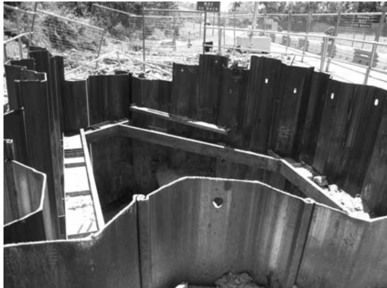
Figure 4.5 A small enclosure with steel sheet piles for an excavation work (Courtesy of N. Sivakugan, James Cook University, Australia)
